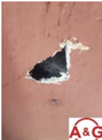
Fibras sueltas (borra de amianto)
